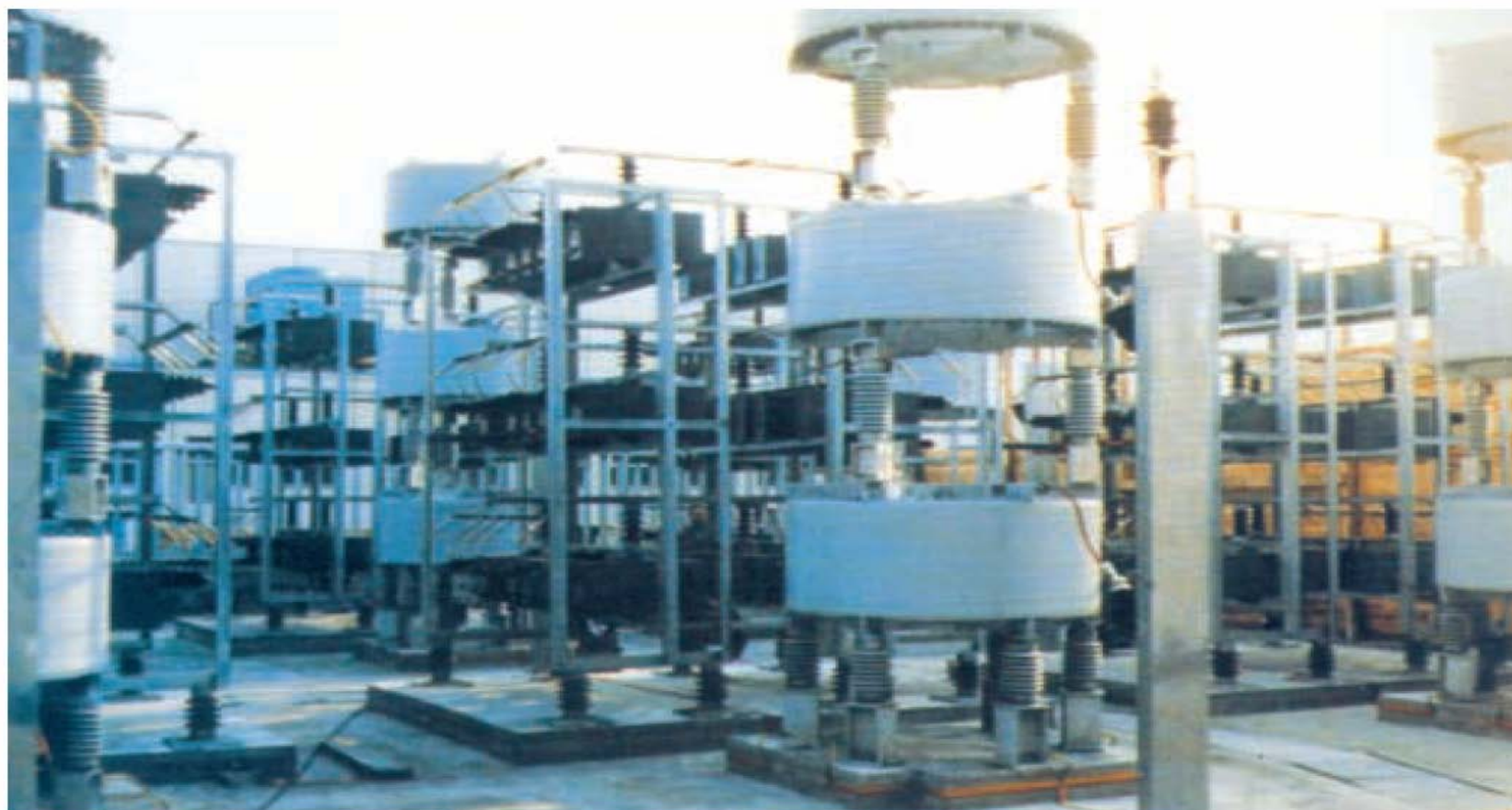
2 x 19,5 MVAR - 22,74 KV - 3rd - 4th harmonics
